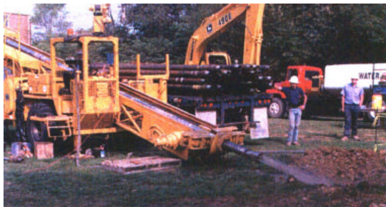
The second shot begins on the Alexandria side of the Potomac crossing. The midi-sized drill rig completed the more than 2,200-ft bore.
