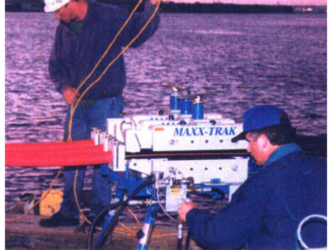
Arnco's A1 Crandall, product manager for placement equipment, adjusts the barge-mounted duct pusher for the insertion of the triple innerduct.
