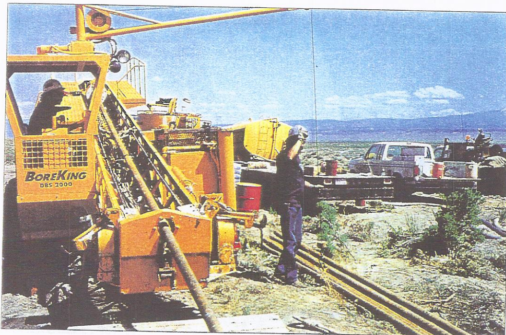
An Ardco BoreKing played an important role in the construction of a new cable conduit in the western U.S. Boring was typically through very difficult soil conditions. Another BoreKing and a Ditch Witch Jet Trak were also used on the project.
