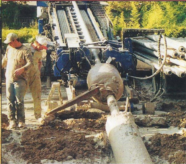
(far left) The drill rig was set up on one side of the river and made a pilot bore under the river bottom to the opposite side.
